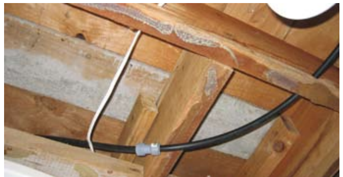
Temporary fix to pipe in ceiling. Leaks caused the ceiling in this room to collapse.
