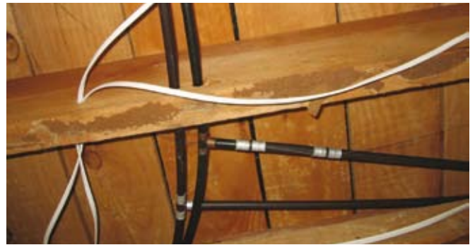
Earlier repairs had already been made to these pipes but they failed again
