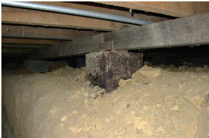
Start with the piles – in situ concrete piles cast in kerosene tins can still be found.
