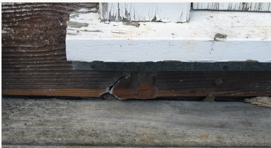
Insufficient gap between cladding and decking.
