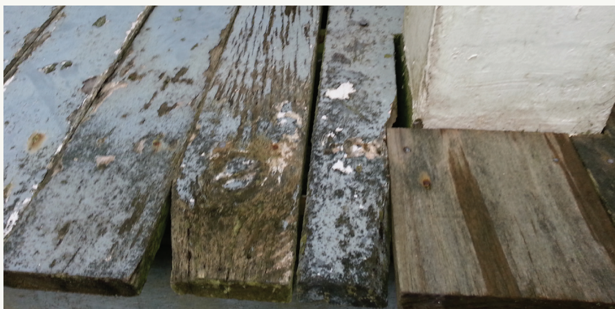
Rotten deck boards.
