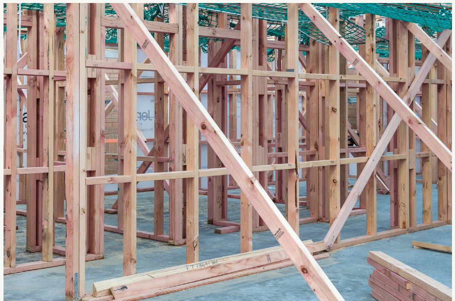
Use of dwangs or nogs (horizontal blocking timber) has changed over time.
