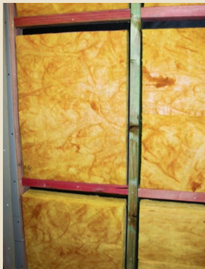
Wall in test with larger gaps around the edges of the insulation.
