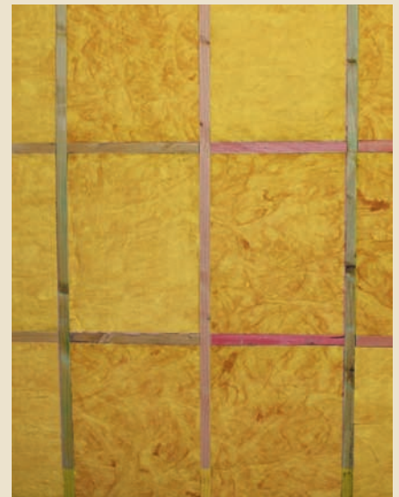
Properly fitted wall insulation in test with no gaps around the edges of the insulation.
