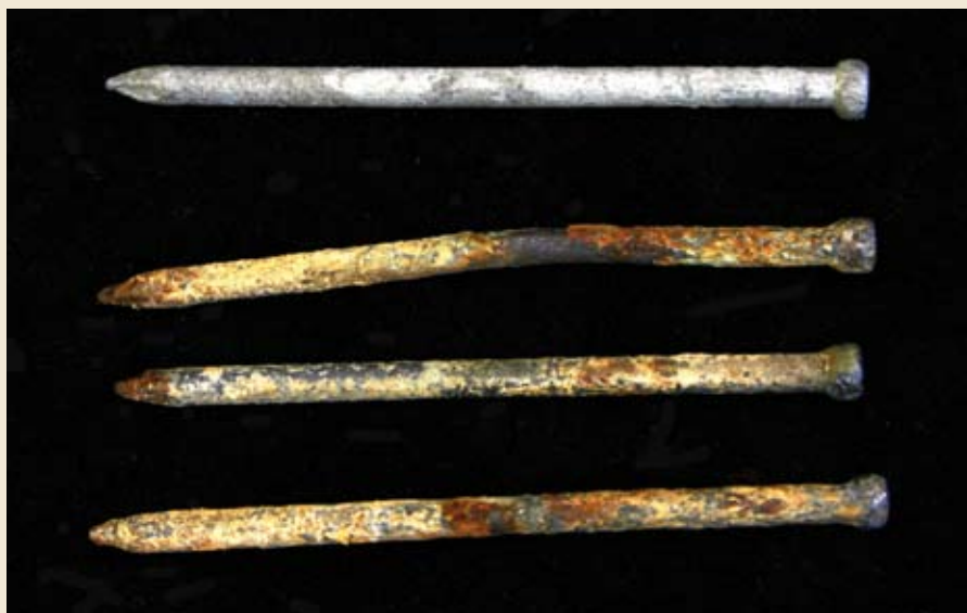
Hot-dipped galvanised nails may not last as long as expected in CuAz- or ACQ-treated timber. Lower three nails shown after 7 years of ACQ exposure in rural Auckland's corrosion zone 1.
