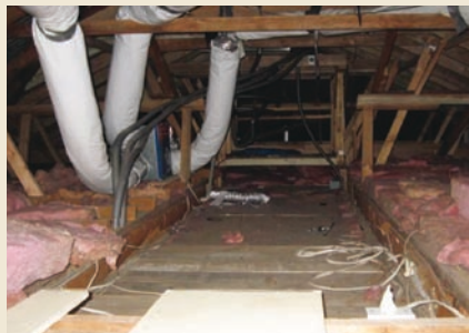
Gaps can be seen beneath the heat recovery ventilation system.
