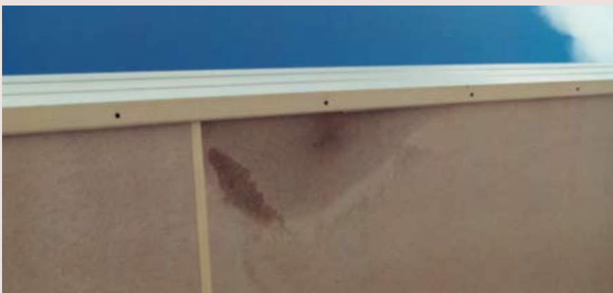
Looking up at the underside of the soffit and concealed guttering with drainage holes. Water staining is visible.
