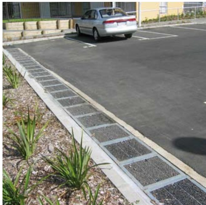
Permeable paving system for stormwater.
