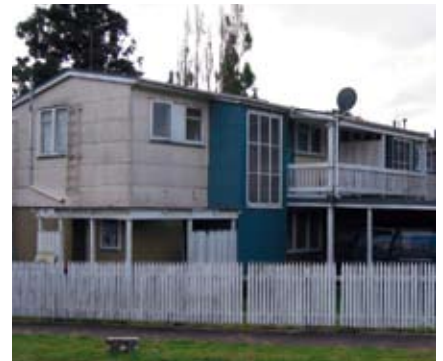
The old 1960s State housing at Talbot Park was in need of upgrading.
