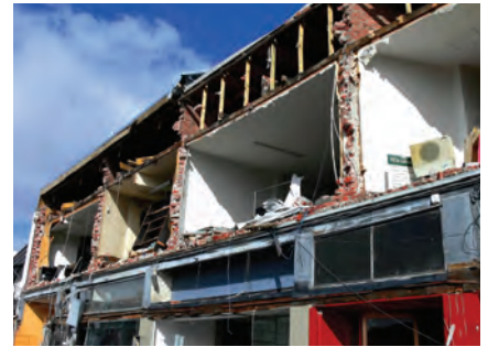
Figure 5: Out-of-plane failure of second storey parapet and façade.
