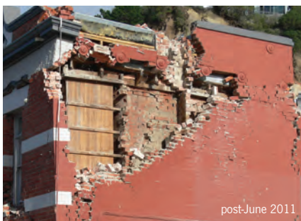
Figure 4: Sequence of damage to a wall following the series of earthquake events.
