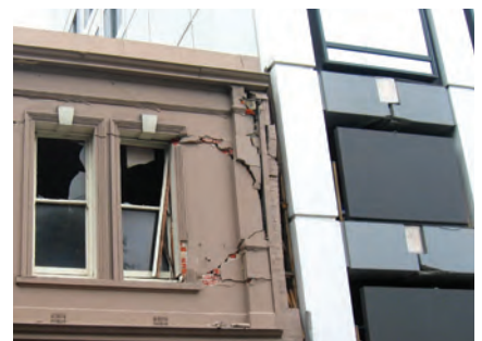
Figure 7: Pounding between two buildings causing diagonal shear cracking in URM building.
