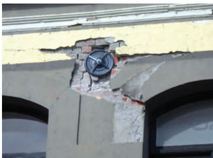
Figure 1: Punching shear failure of roof rafter anchor plates. This type of damage was widespread.
