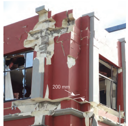
Figure 6: The corner detail shows this upper storey has slid by 200 mm.
