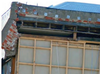
Figure 2: Row of successful wall-diaphragm anchors, despite the wall failure beneath.
