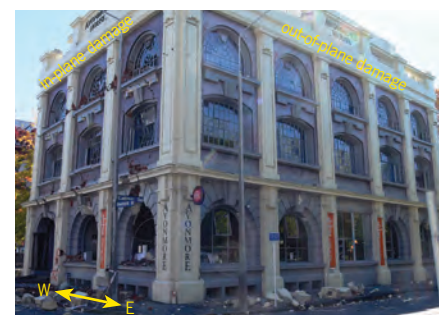
Figure 3: Looking at the southeast corner of this building, the in-plane shear cracking is only visible on the south face indicating the predominant shaking was east–west.
