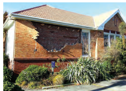
Figure 11: Although this URM had been retrofitted with high-strength twisted stainless steel ties, it failed during the 13 June 2011 earthquake.
