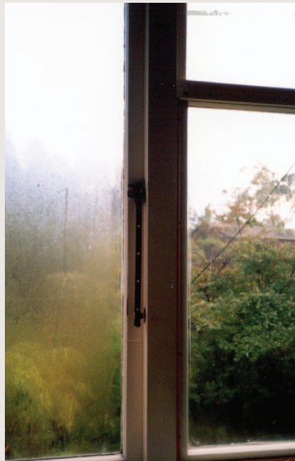
Figure 1: Internal condensation forms on the cold single-glazed pane on the left but not on the warmer doubled-glazed pane on the right.
