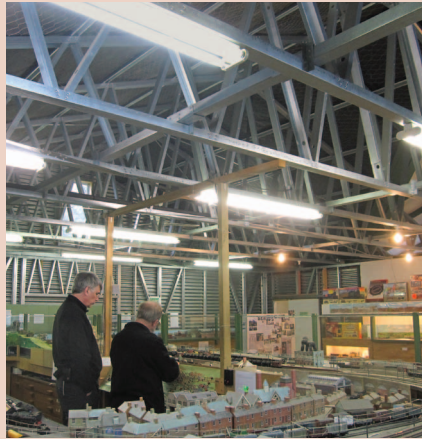
A very early light steel frame building built in the mid 1990s.
