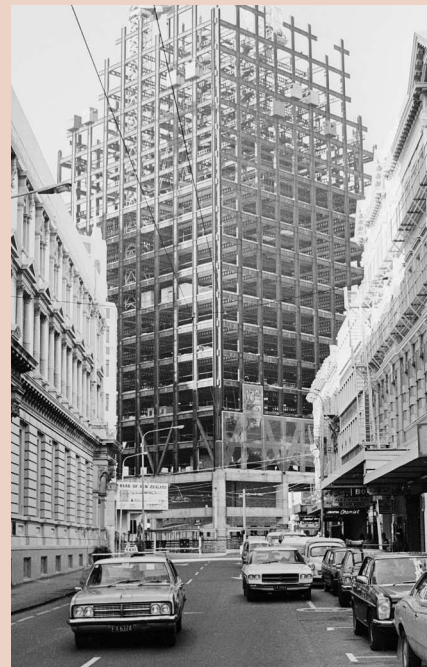
The steel frame of the State Insurance Tower, Wellington (known as the Bank of New Zealand Tower up until 1998) in 1979. (Photo from Alexander Turnbull Library, Dominion Post Collection (PAColl-7327). Reference: EP/1979/2632/10. Photograph by Ron Fox.)
