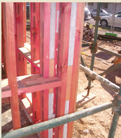
Figure 1: Insulation needs to be installed beforehand in all areas that cannot be accessed after the building wrap is installed. In this case, the insulation is grey.
