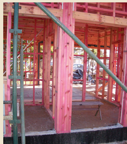
Figure 2: The stud to stud butt joint (thermal bridge) common on most sites today, where framing is constructed off-site.
