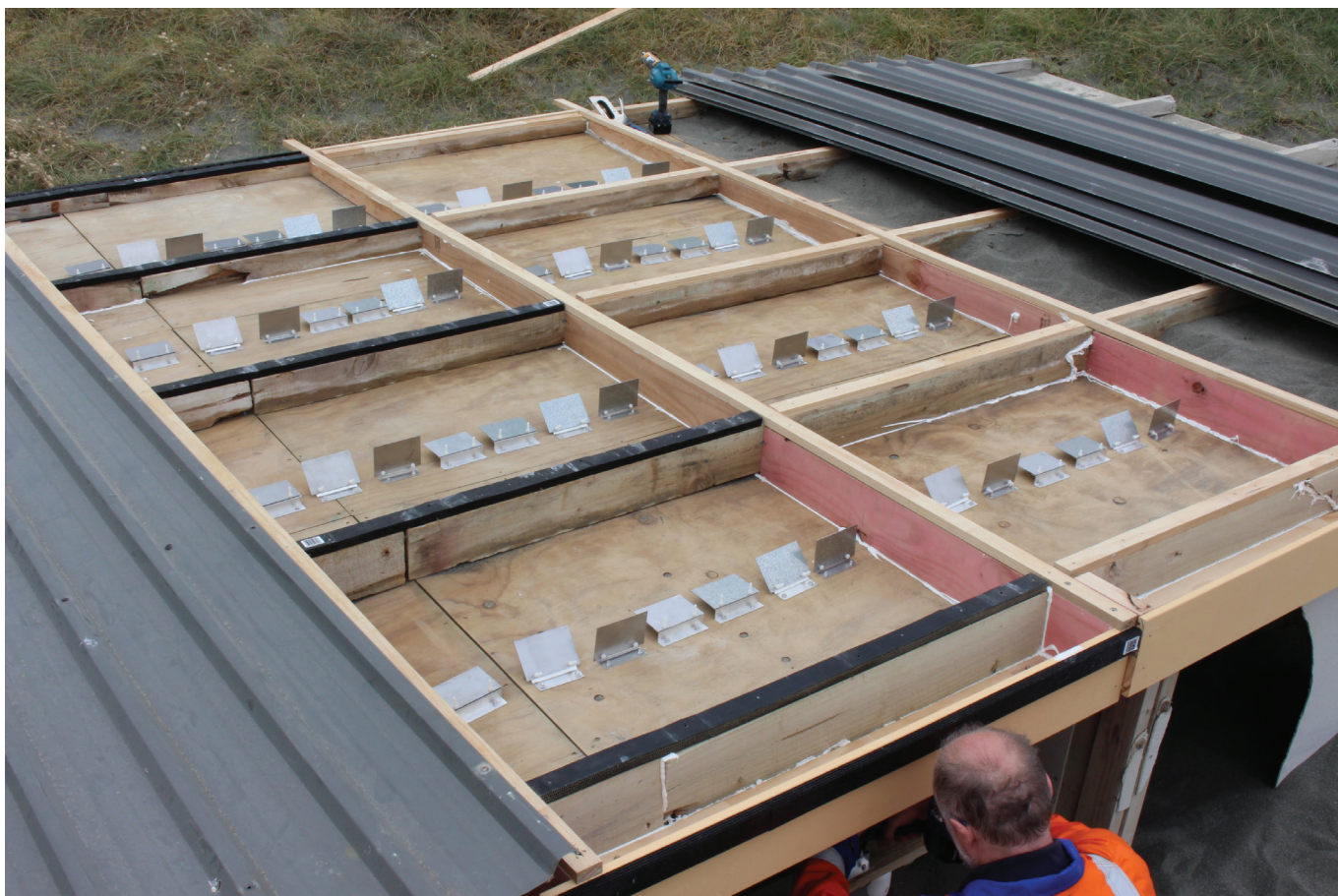
Figure 1: Mild steel and galvanised samples were mounted inside the vented and unvented roof areas at different angles – vertically, horizontally and at 45° to vertical.
