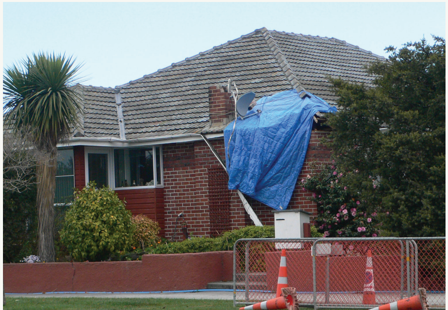
A chimney that collapsed in the Christchurch earthquakes.
