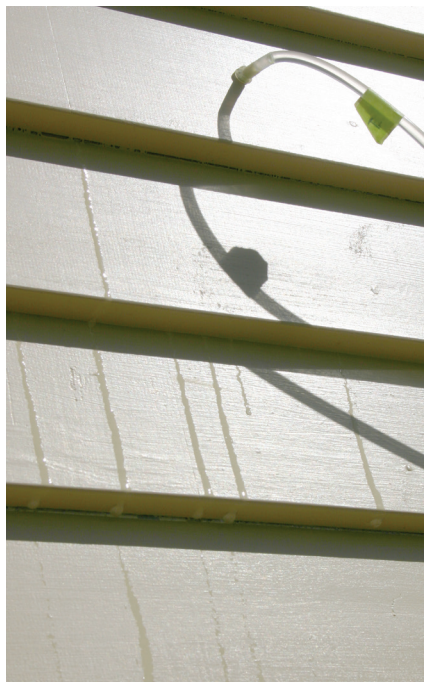
Figure 3: Water draining from laps visible on weatherboard face in test sample.
