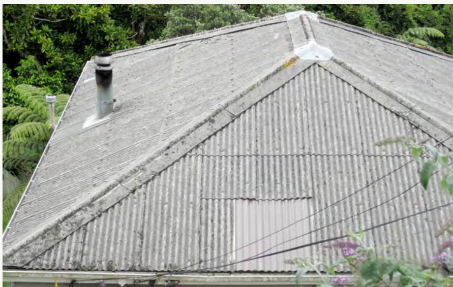
Corrugated asbestos roof.
