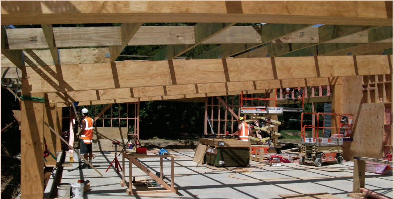
The refurbishment of the BRANZ site includes construction of the new Nikau building – a single-storey, monopitched office space constructed using a post-tensioned LVL portal frame that spans the width of the structure.
