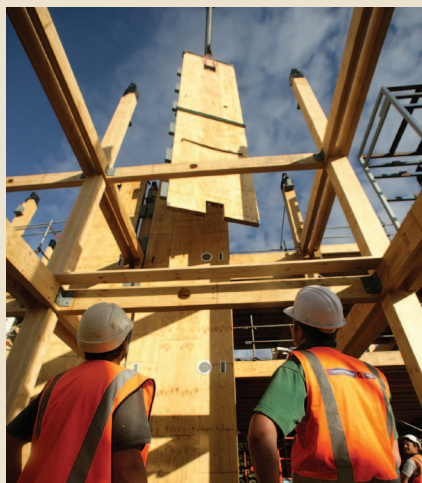
Nelson Marlborough Institute of Technology's new Arts and Media building makes extensive use of locally sourced materials, including these laminated veneer lumber beams, which form the primary structure of the building.
