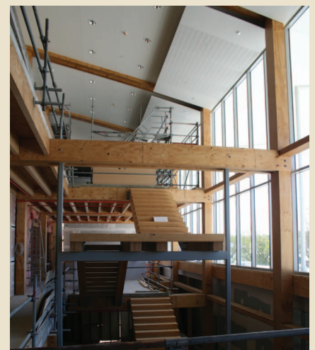
As construction progressed, it became clear that the building's extensive use of exposed timber would offer an aesthetically pleasing interior environment.
