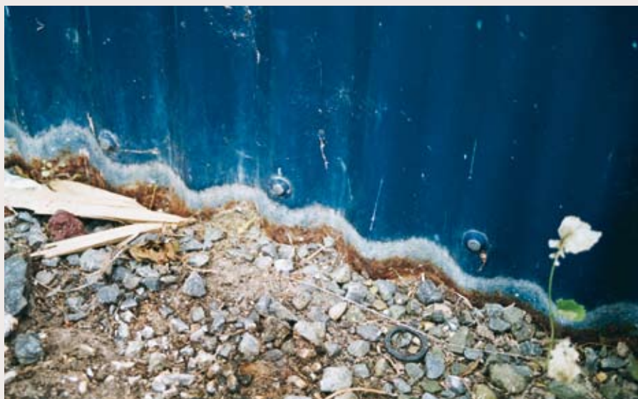
This photo of a 1990s house close to the coast shows what happens when the cladding clearance is insufficient. Source: 2005 BRANZ House Condition Survey.
