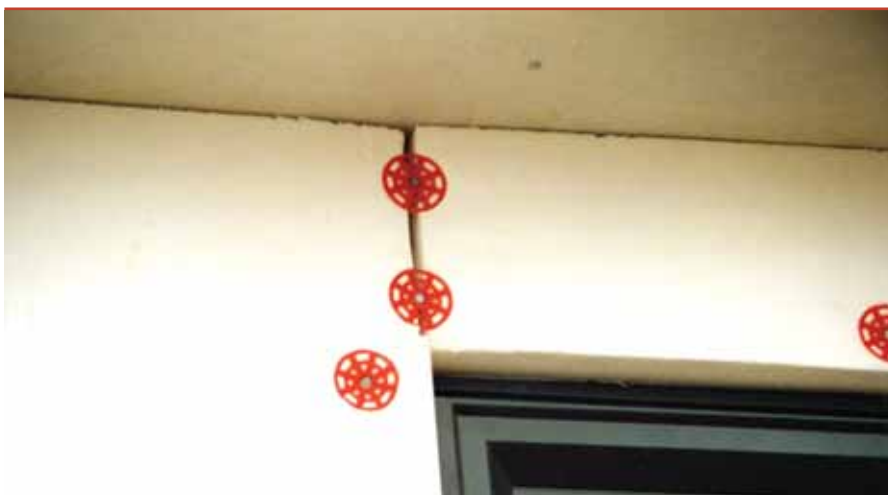
Figure 2: If gaps between the polystyrene boards are filled with the base coat they create a thermal bridge. Cracks may also appear along the line of the joint because of differential expansion in the base coat when temperatures rise.
