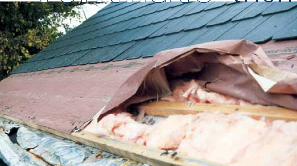
| A roof with a moisture problem, but is lack of ventilation the cause?
