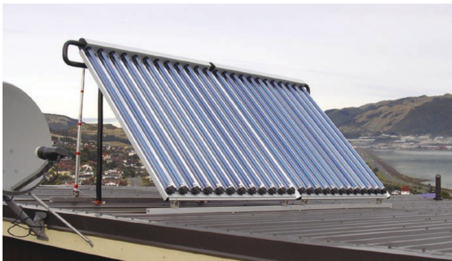
Correct positioning is essential to get good performance from a solar collector.
