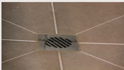
It is important to specify a floor waste to all bathrooms as overflows will occur.
