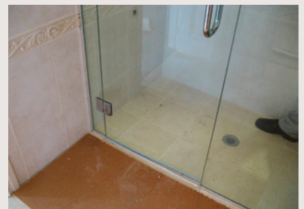
Ensure the threshold at the door is high enough to contain the water within the shower and that the floor has a slope to the outlet.
