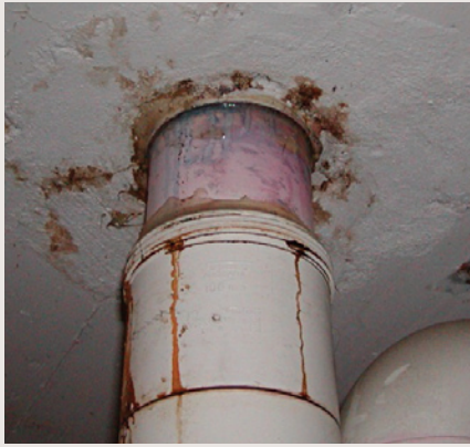
Waste pipe with no seal.
