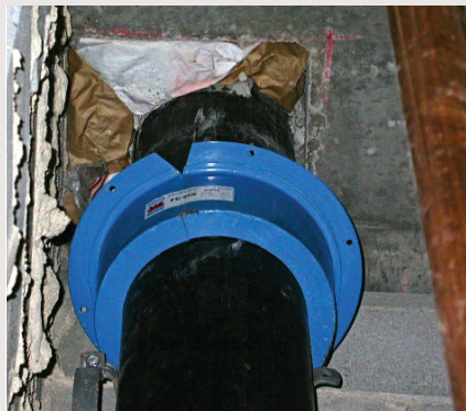
An example of inappropriate packing of the aperture.
