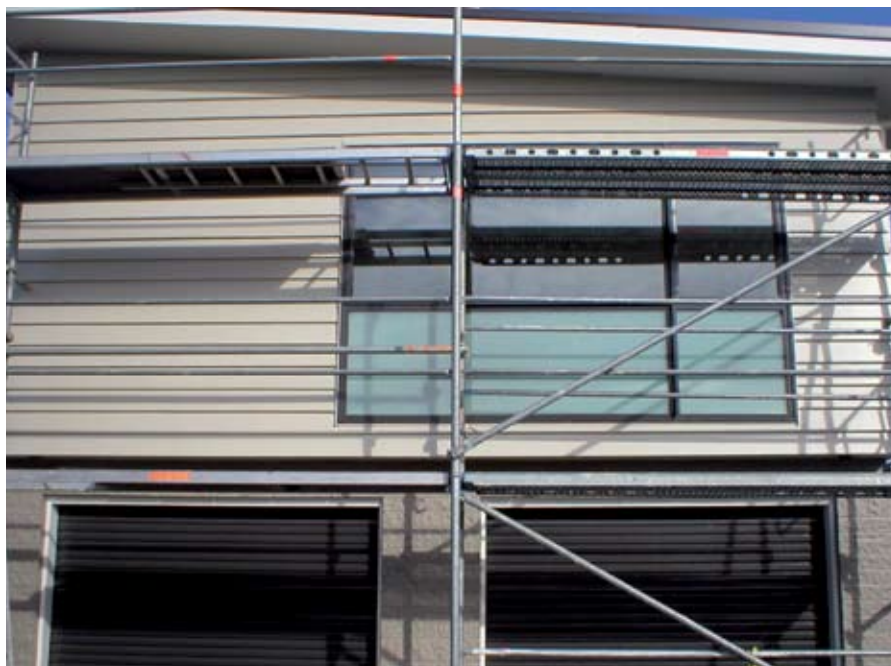
A large replacement window with IGUs being installed into an existing house.
