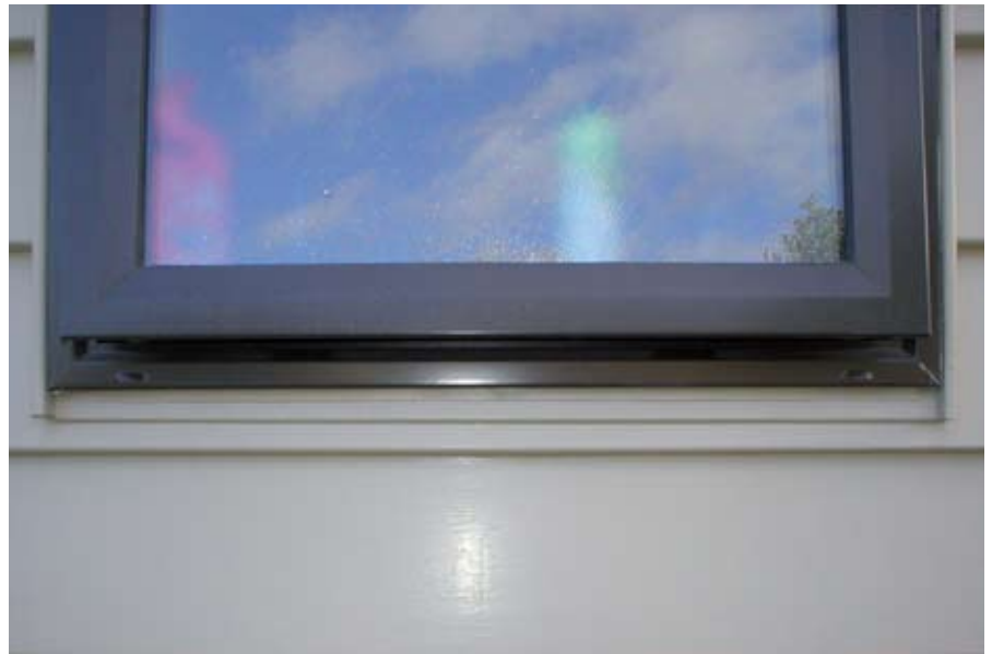
Installing replacement glazing into an existing window frame was quick and caused little disruption.
