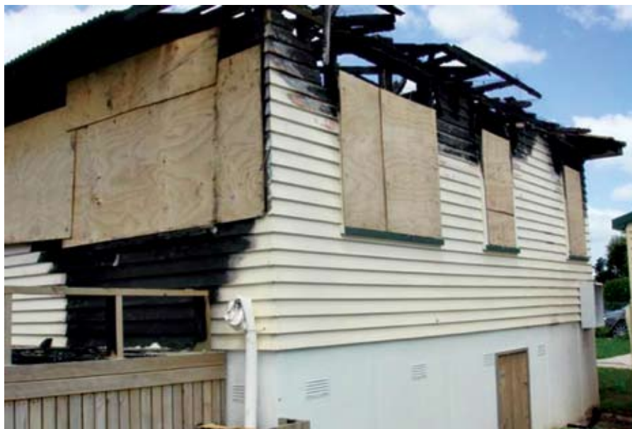
Plywood is used to secure the house from vandalism.
