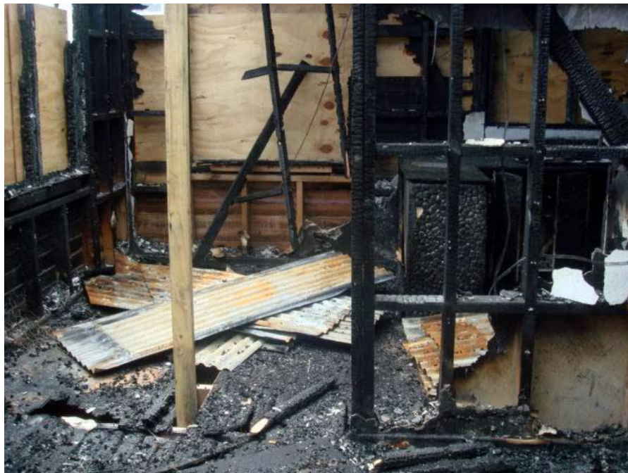
Some framing is more damaged than the rest. Up to 3 mm can be scraped off the timber before it must be replaced. Stud is holding up temporary roof frame for canopy. Floor covering is damaged but not joists.
