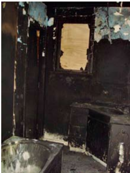
A fire-damaged bathroom. The bath is likely etched from the soot and will need replacing as will the vanity, ceiling, wall and floor linings and internal door.
