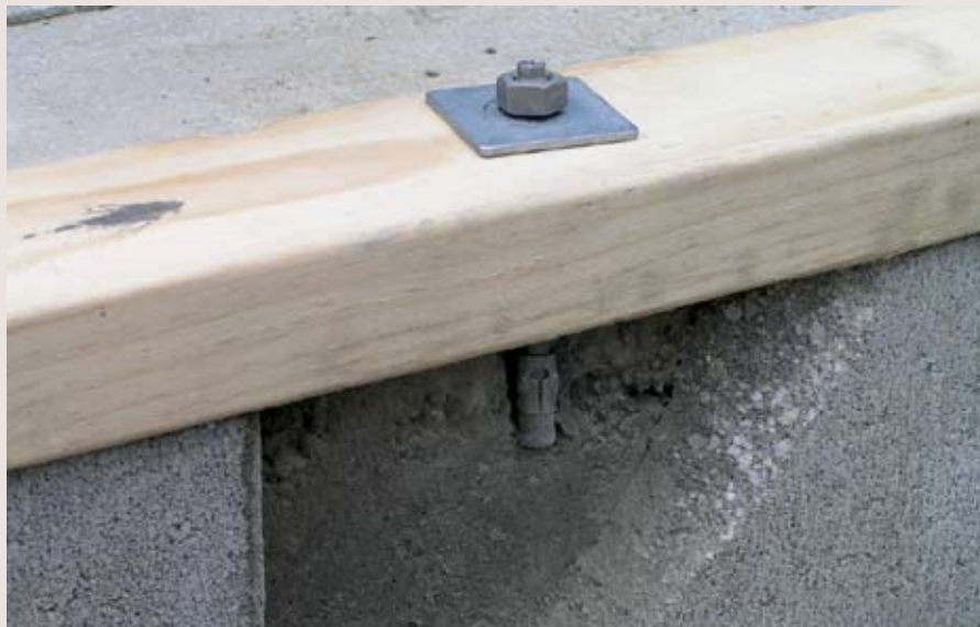
Remedial work can not satisfactorily fix this problem.
