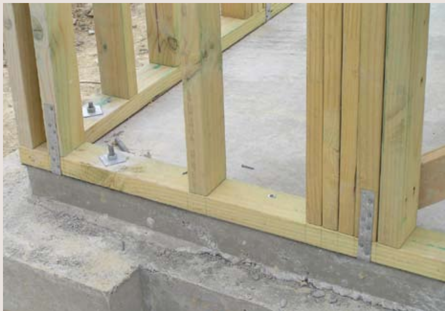
The importance of bottom plate anchors is clearly not understood on this job with one bolt missing.
