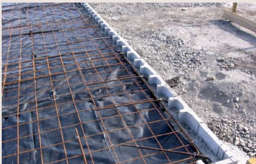
Providing an adequate fixing for external bottom plates will not be easy for this slab.
