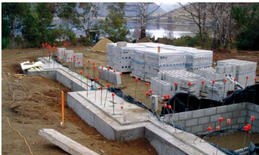
Figure 4: The foundations are poured and the construction of the passive cellar can be seen, which provides cooling for the house.
